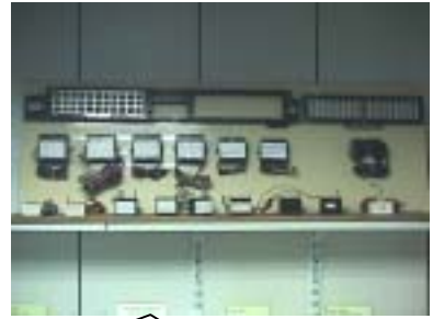
High voltage generators
